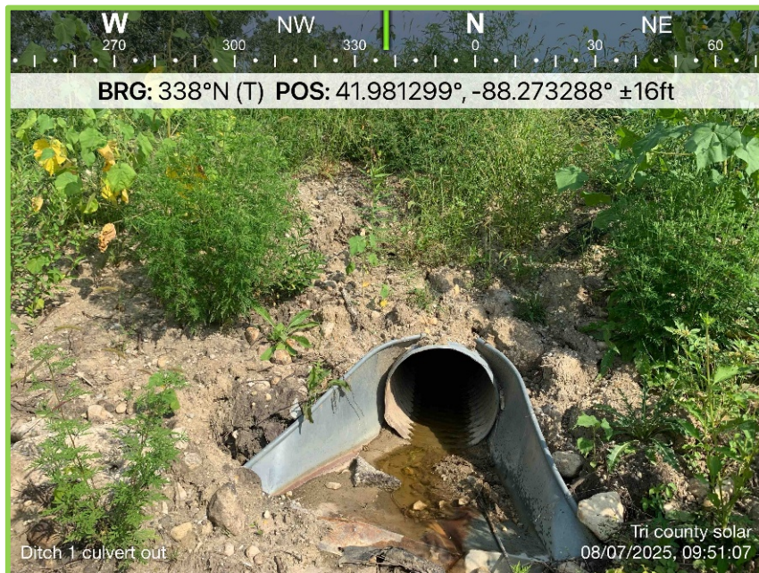
Culvert Out where Ditch 1 begins
